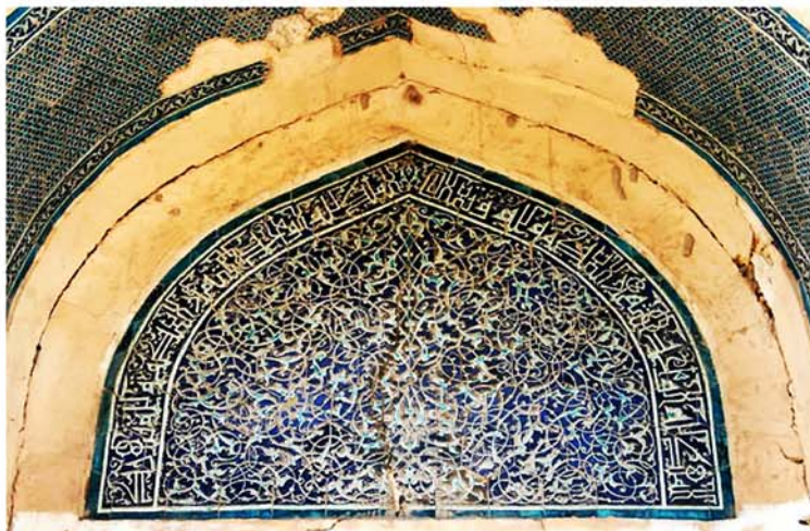
17 Underglaze-painted low-relief tilework of tympanum over door, Mausoleum of Najm al-Dīn Kubrā, Urgench, Khwarazm, Turkmenistan
