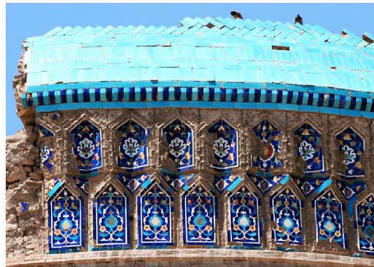
49 Section of the collapsed turquoise, ribbed outer roof shell of the Mausoleum of Tura Beg Khanum, Urgench, Khwarazm, Turkmenistan
